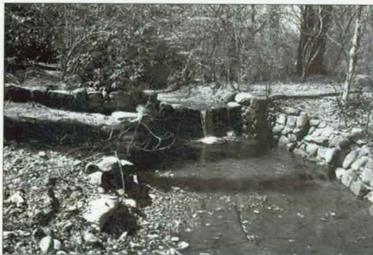
Figure 154 Old Water Wheel Falls as seen after the south bank wingwall was rebuilt, April 1, 1997. NCR, Photo Archive, DOP 2-1a.
