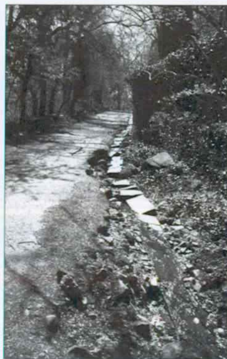
Figure 191 Slate slab gutter with stone rill along Lovers' Lane, August 1997. NCR, Photo Archive, DOP 40-13.
