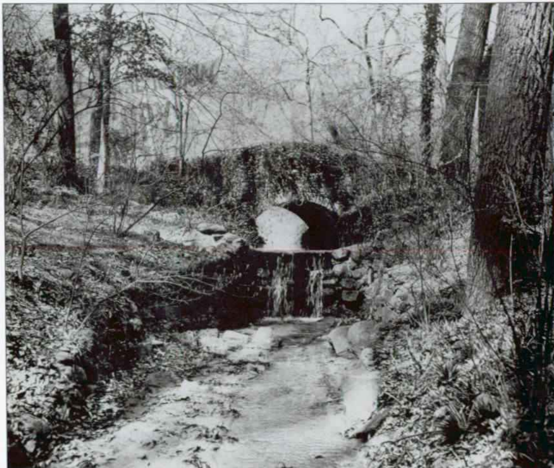
Figure 160 English ivy was allowed to grow on the stone bridge. April 12, 1963. MRC, Photo Archive, #96
