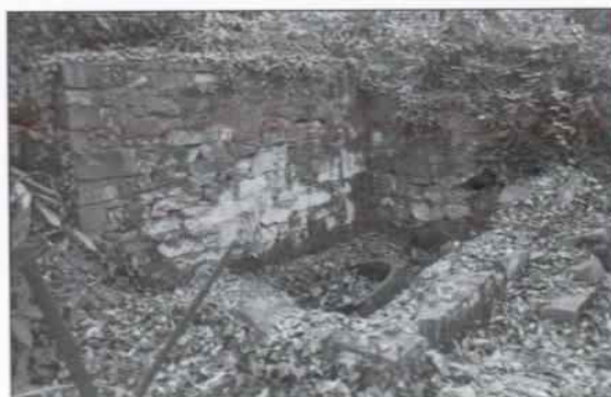
Figure 54 Rusted broken parts from the old water wheel are laying beside the Old Pump House, December 1998. NCR, Photo Archive, DOP 48-22.
