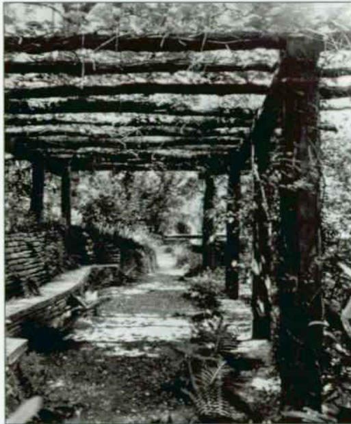
Figure 133 Clumps of ferns grow in pockets along the back of the Stream Arbor wall and a tangle vines grows on the arbor, c. 1935. DOSLA, Photo Archive, #13.4.
