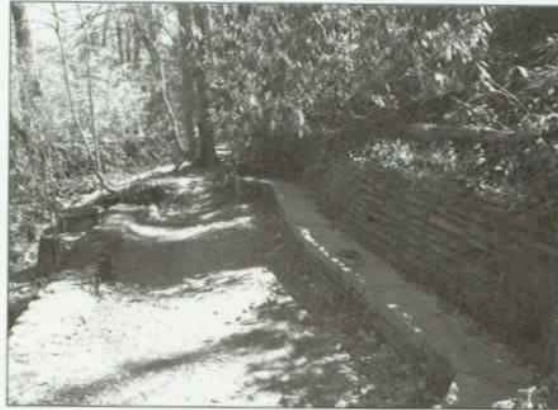
Figure 55 Many of the original flagstones that were laid beside the cedar channel, have been displaced or lost, April 1, 1997. NCR, Photo Archive, DOP 2-3a.
